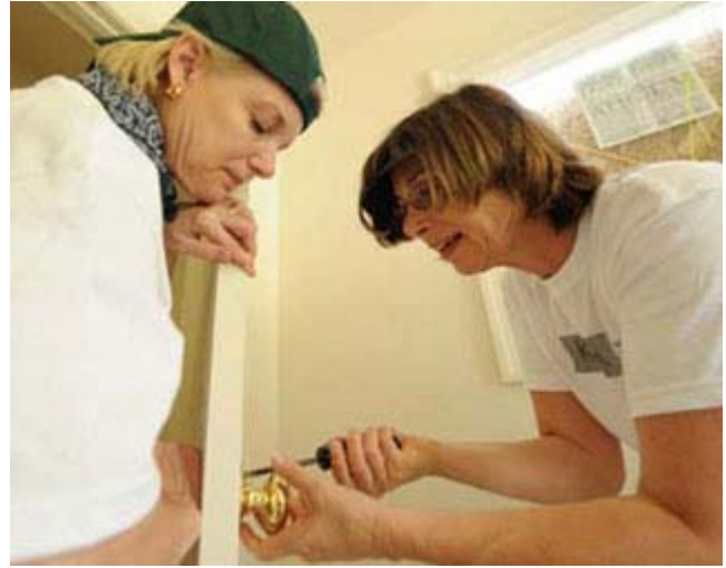
Code Council and Foundation Board member Barbara Koffron (left) and Karen LaTorra, wife of ICC Board member John LaTorra, install door hardware during the Habitat for Humanity work project held during 2008 Building Safety Week festivities.
